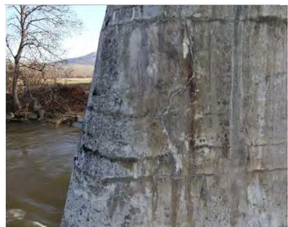
2° Example of pathologies found in buildings
