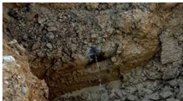
Leakage of a pipe
