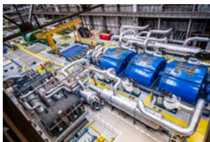
Machine room of the Tricastin Nuclear Plant
