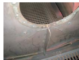
Picture of cracked divider
