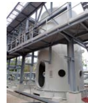
S605 filter installed in the MVR unit
