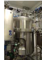
C401 pressure vessel on customer site
