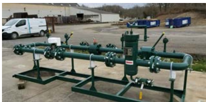
Marckolsheim - DN100 gas line substation
